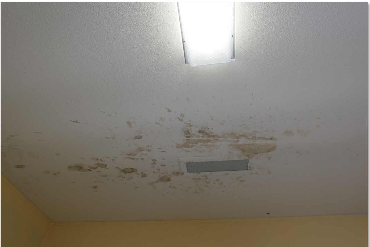
Photo 8: Old stains were visible.
