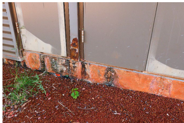
Photo 7: Water damage to concrete pad
