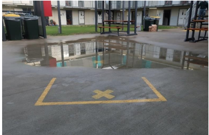
Photo 5: Pooling water in Unit 6
